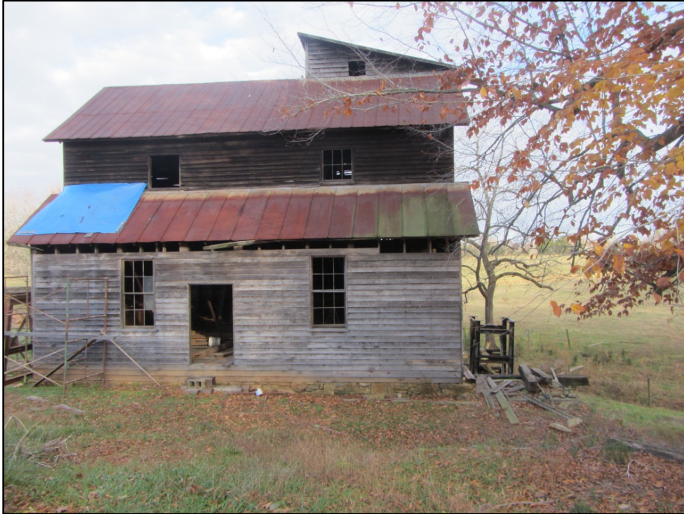
Figure 8. Ward Mill (AM 457), west elevation, looking east from Coble Mill Road. Door and window panes have been removed.
