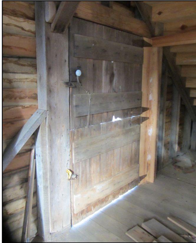
Figure 17. Ward Mill (AM 457), interior view of door (not original) on north elevation.
