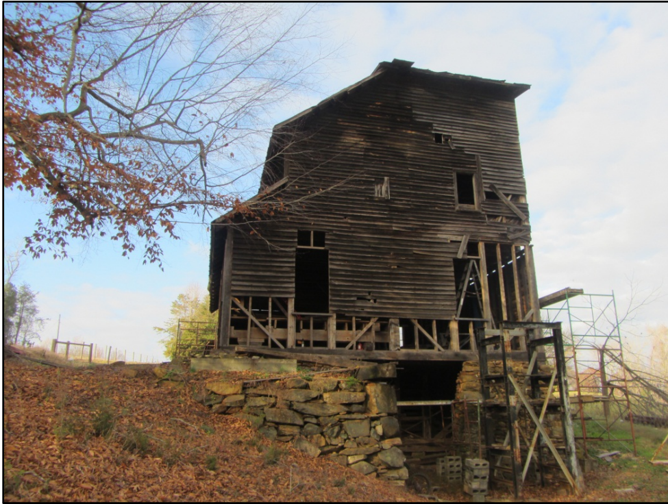
Figure 5. Ward Mill (AM 457), south elevation and foundation, looking north from Cane Creek.
