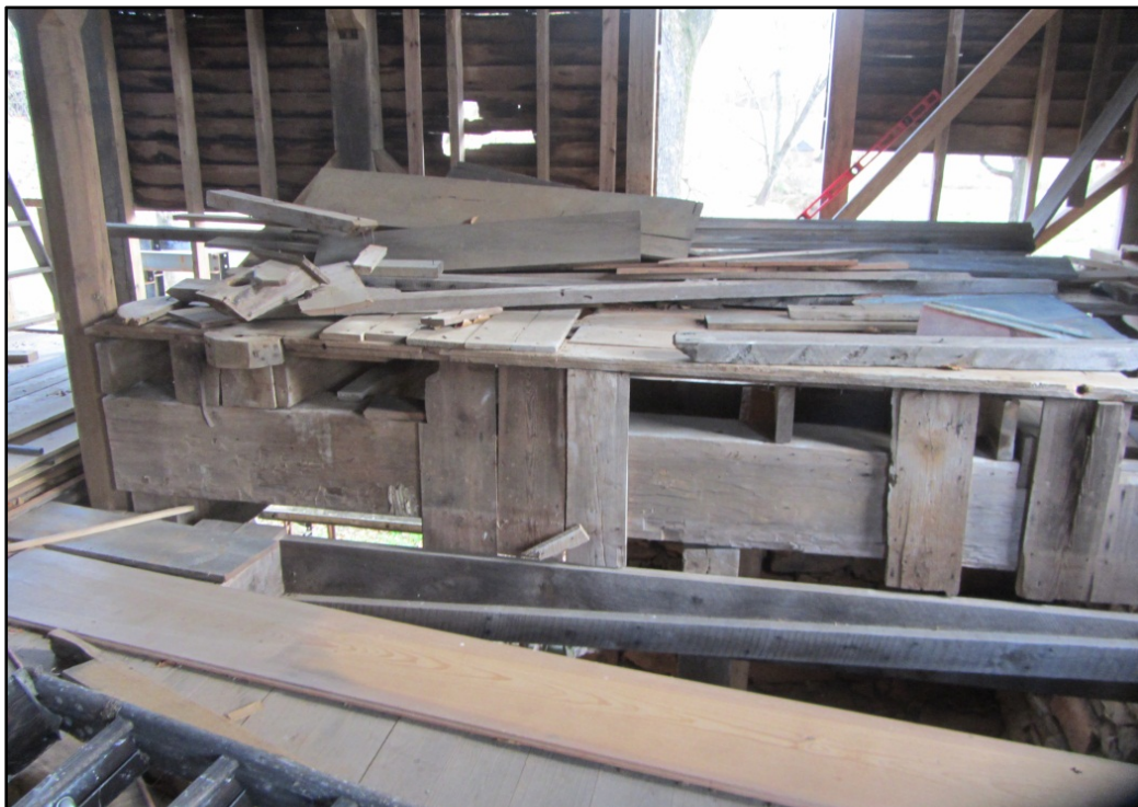
Figure 16. Ward Mill (AM 457), first-floor interior view, detail of box for mill machinery being repaired.
