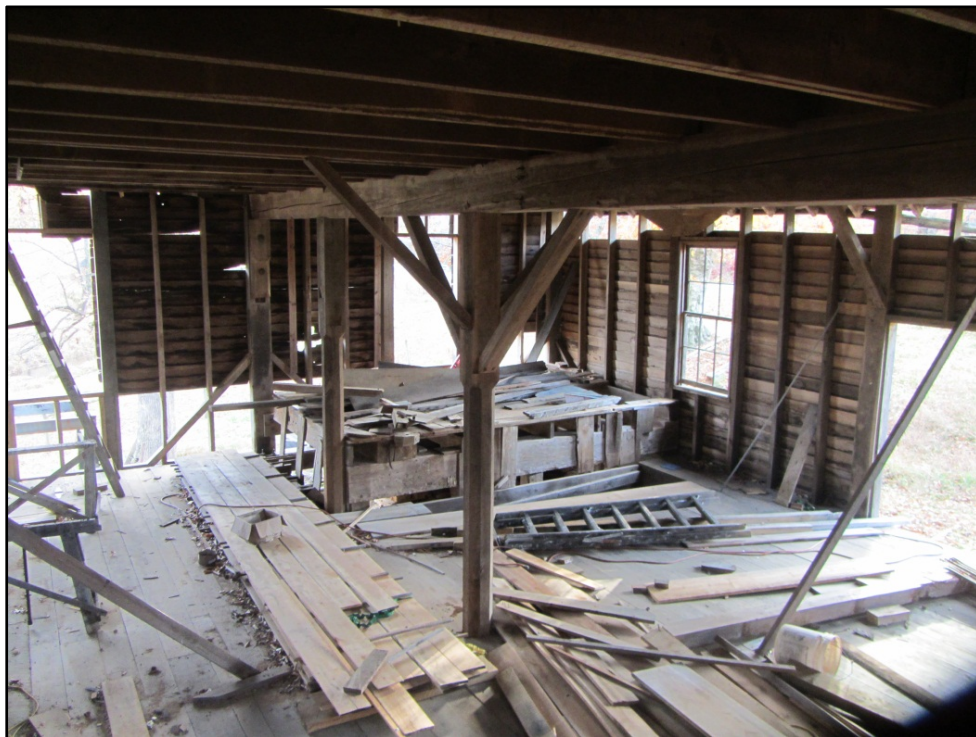
Figure 22. Ward Mill (AM 457), second-floor interior view, looking northeast toward staircase, showing replaced floors, wall studs, lathe, and window sash with removed panes.
