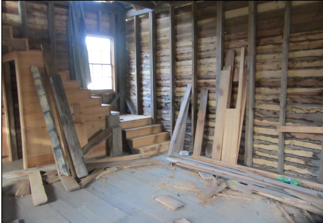
Figure 14. Ward Mill (AM 457), first-floor interior view, looking northeast toward rebuilt staircase. Walls and floors in process of being replaced or repaired.
