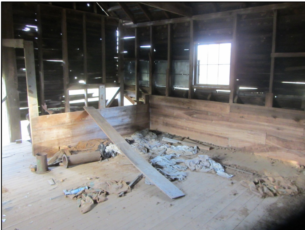
Figure 20. Ward Mill (AM 457), interior second-floor view looking toward staircase and northeast building corner, showing replaced floors, exposed walls studs, and sash with panes removed.
