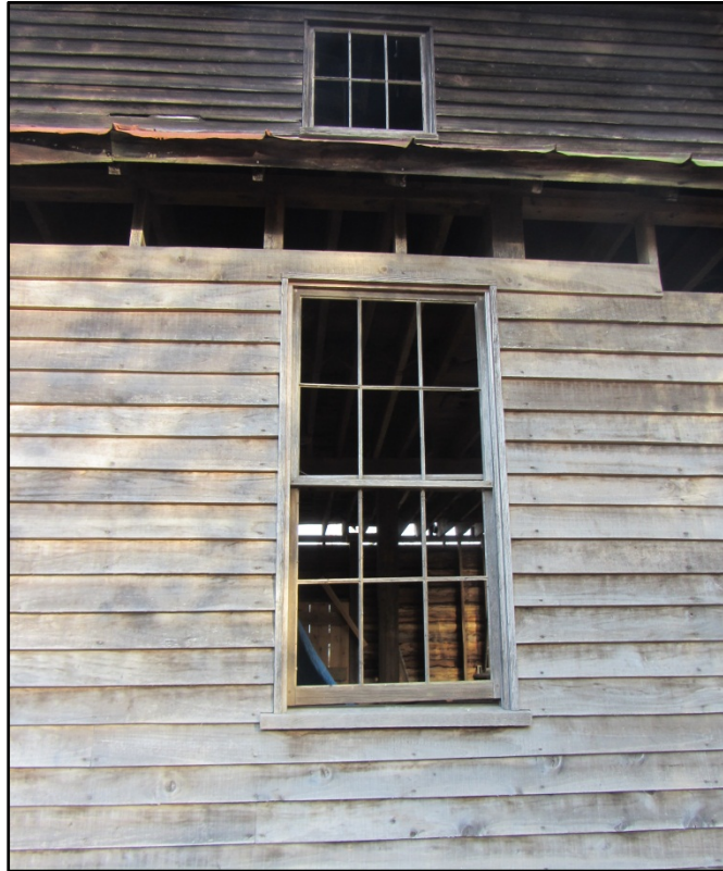
Figure 9. Ward Mill (AM 457), detail of windows on west elevation, looking east. Window panes have been removed.
