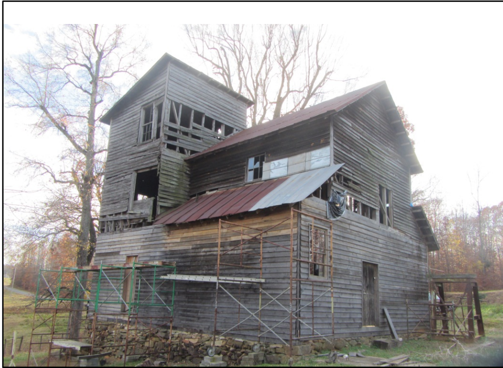
Figure 13. Ward Mill (AM 457), northeast corner of mill, looking southwest. Siding and windows in process of being replaced.
