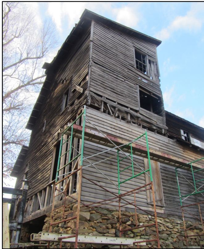
Figure 12. Ward Mill (AM 457), southeast corner with detail of rebuilt foundation and replaced siding, looking northwest.
