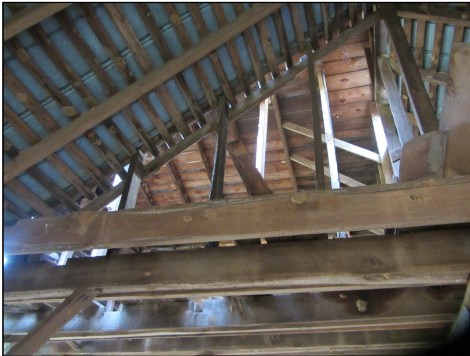
Figure 18. Ward Mill (AM 457), view of roofing system looking up toward the exposed third floor, showing the replaced roofing members.
