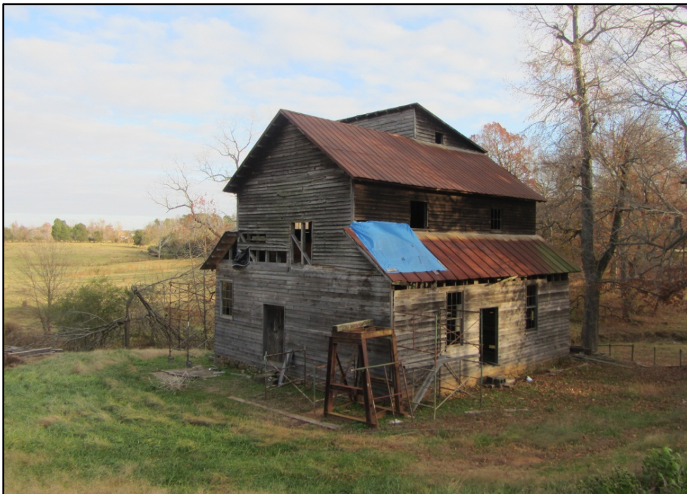
Figure 10. Ward Mill (AM 457), northwest corner of mill, looking southeast from Coble Mill Road. Doors have been removed and some window sash removed entirely.
