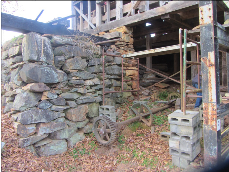
Figure 6. Ward Mill (AM 457), detail of rebuilt foundation and wheel pit, looking northwest.
