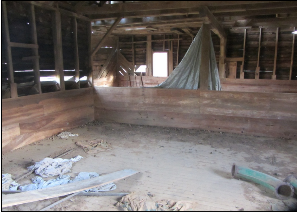
Figure 21. Ward Mill (AM 457), second-floor interior view, looking southwest toward partially rebuilt walls and a partition wall.
