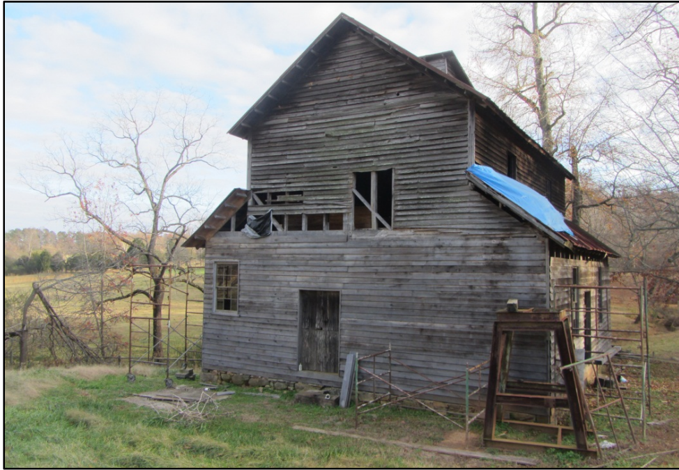
Figure 11. Ward Mill (AM 457), north elevation, looking south/southeast. Siding in process of being repaired or replaced.
