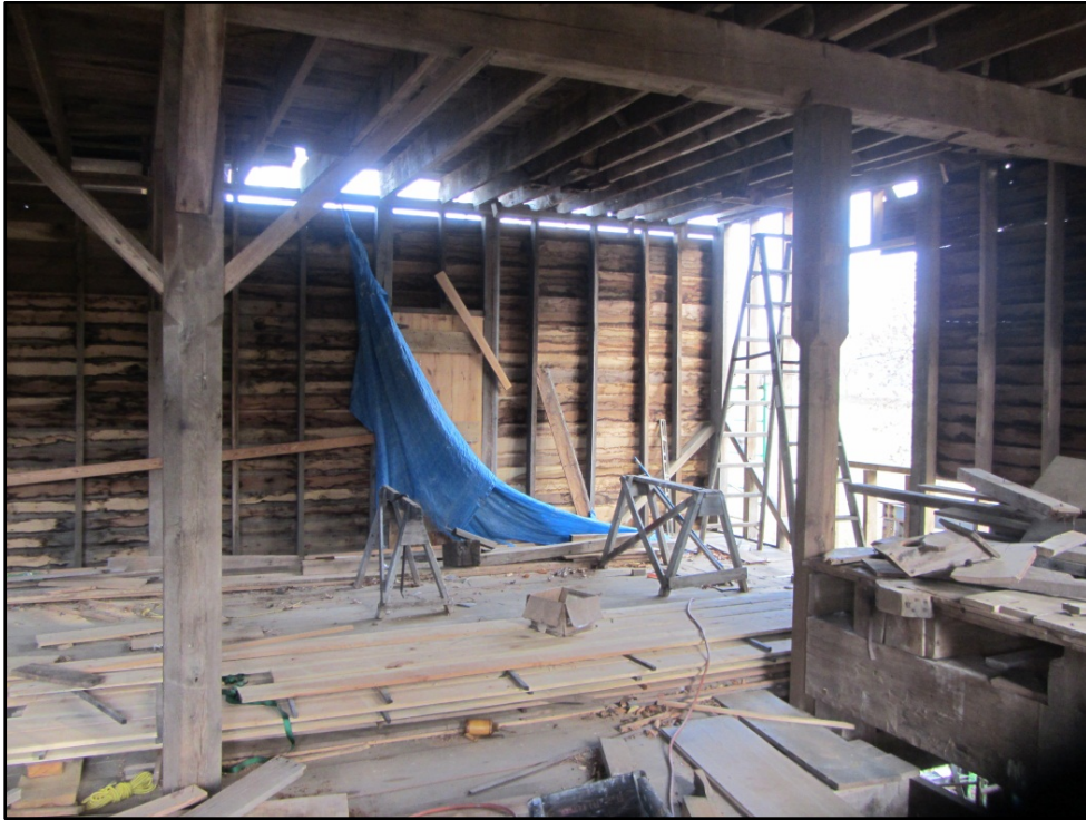
Figure 15. Ward Mill (AM 457), first-floor interior view looking southwest from entrance. Floors being replaced and the wall left open on the south side.
