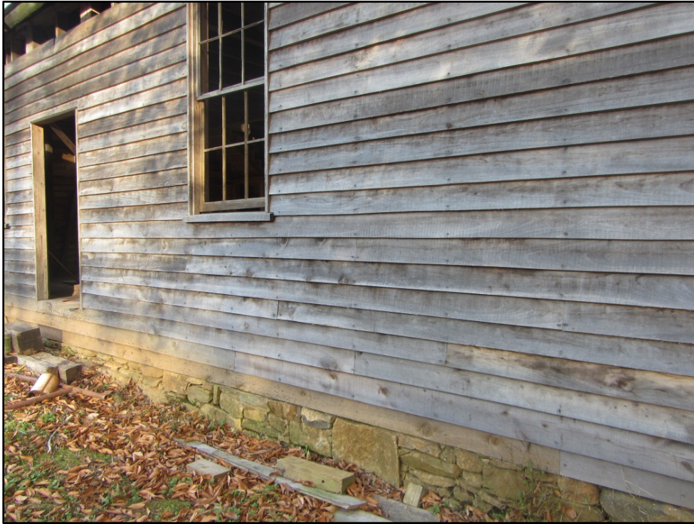
Figure 7. Ward Mill (AM 457), detail of rebuilt coursed stone foundation on west elevation, looking north/northeast.
